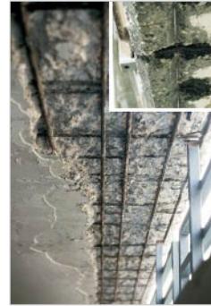
Damage after eight years on the underside of a balcony concrete sheet with no water drip or drip edge at all
