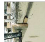
Damage to the concrete sheet of a balcony due to insufficient concrete cover. The repair illustrated where the water drip is reshaped by insertion of a triangular strip retains the weak points and will not be successful in the long term
